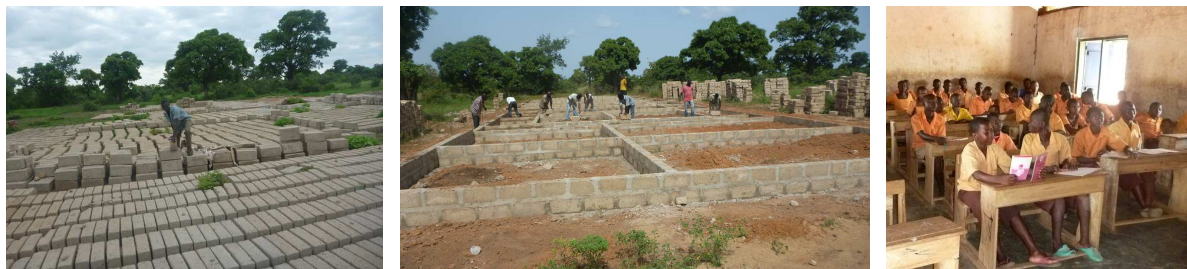
Building of the blocs, Laying of the foundation for the JHS, First students of the new JHS (left to right).
